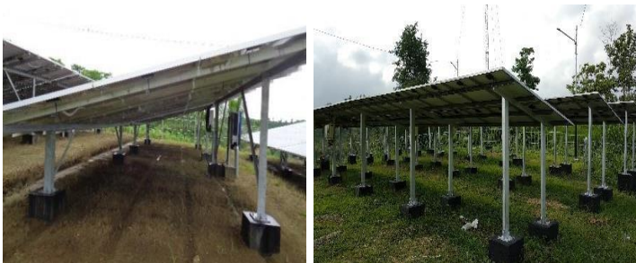
Gambar 9.1 PLTS Ground Mounted
