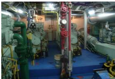
Picture 10.3 : Engine room
